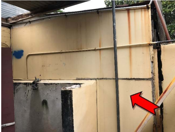
Photo 1. Interior, throughout south elevation, wall – asbestos-containing fibre cement sheeting.
